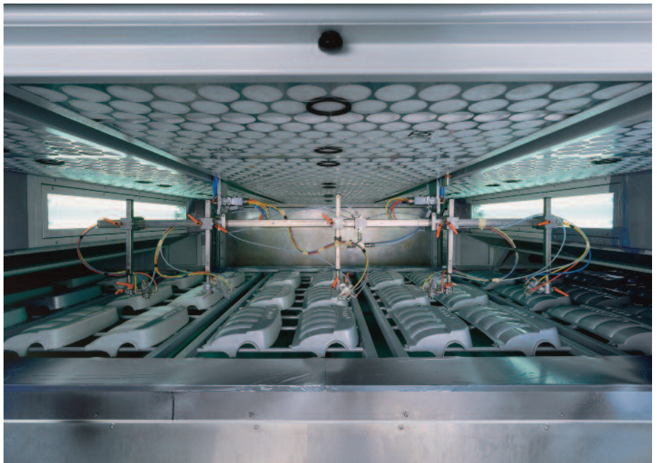
Light fittings of series e192 ... mounted in a paint shop
